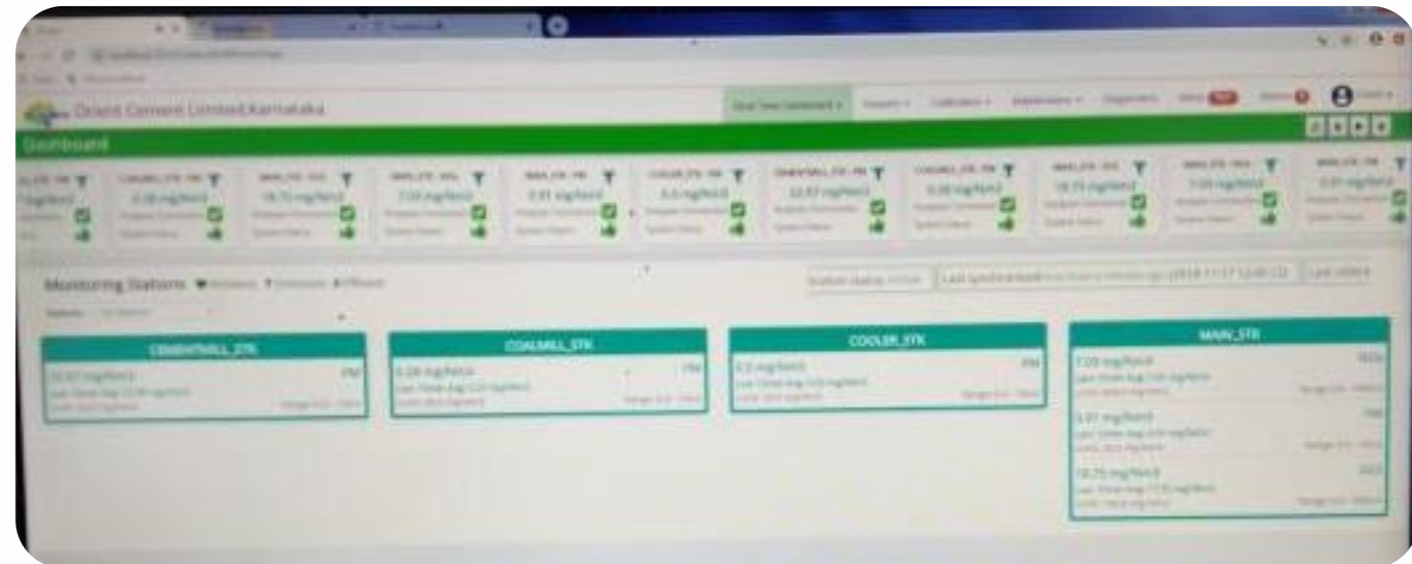
Control Room Display
