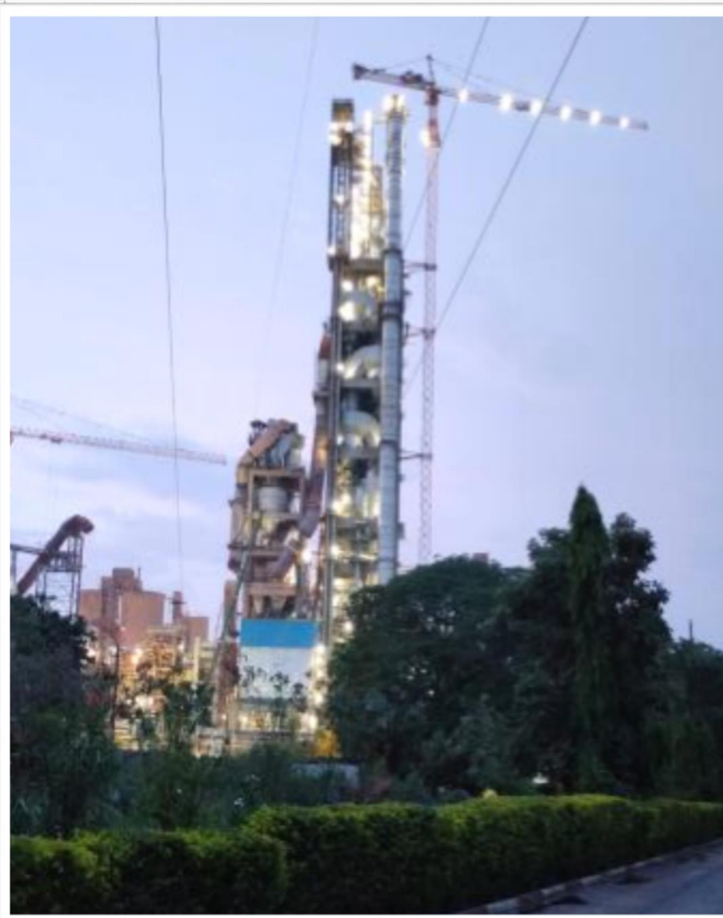
SLC to ILC on ongoing modification with CCX cyclone & Specially design Calciner for AFR utilization
